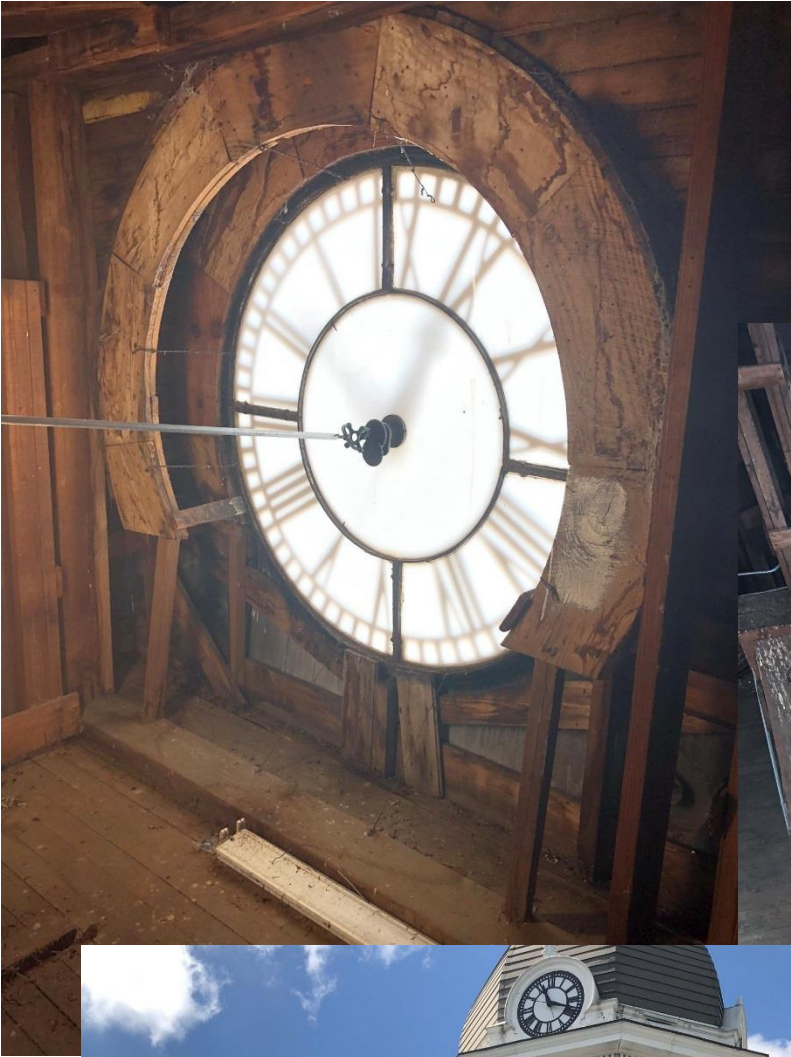
The interior face of the clock shows stains from leaks as does the floor area around the bell and the historic bell itself.
