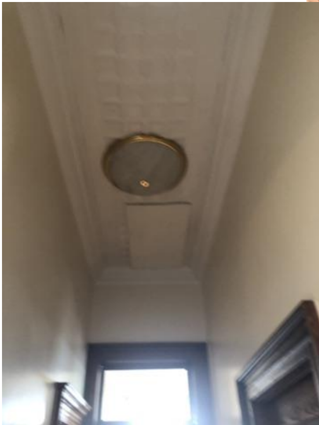
Additional water damage and lighting photos including a glimpse of the fluorescent lighting.
