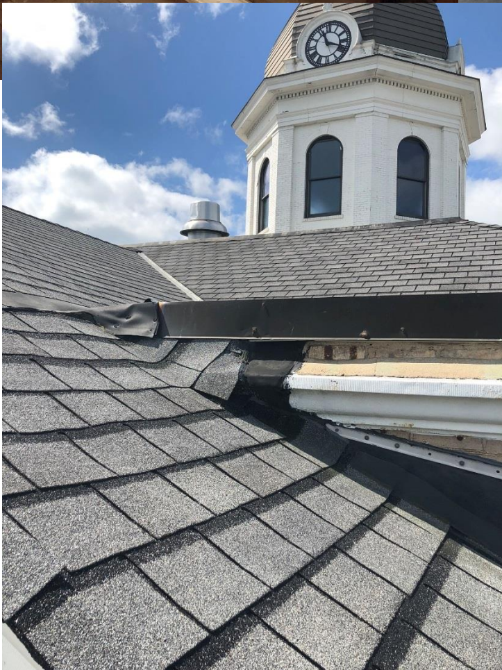
Repairs have been made over the years to address leaks. The photo at left is taken at the transition of the Greene Street Portico onto the main, hipped Courthouse roof.
