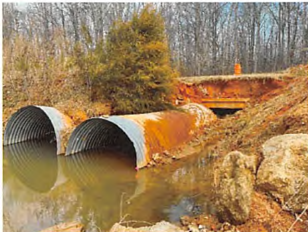
Photo 1. Upstream view of failed culverts.
