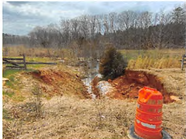
Photo 2. Downstream view of failed culverts.
